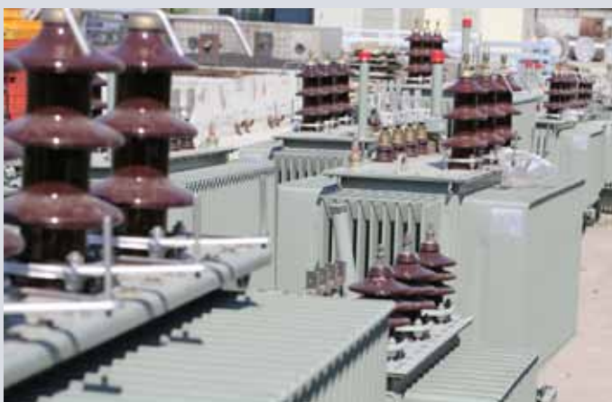
Pole mounted 200kva transformers awaiting inspection
